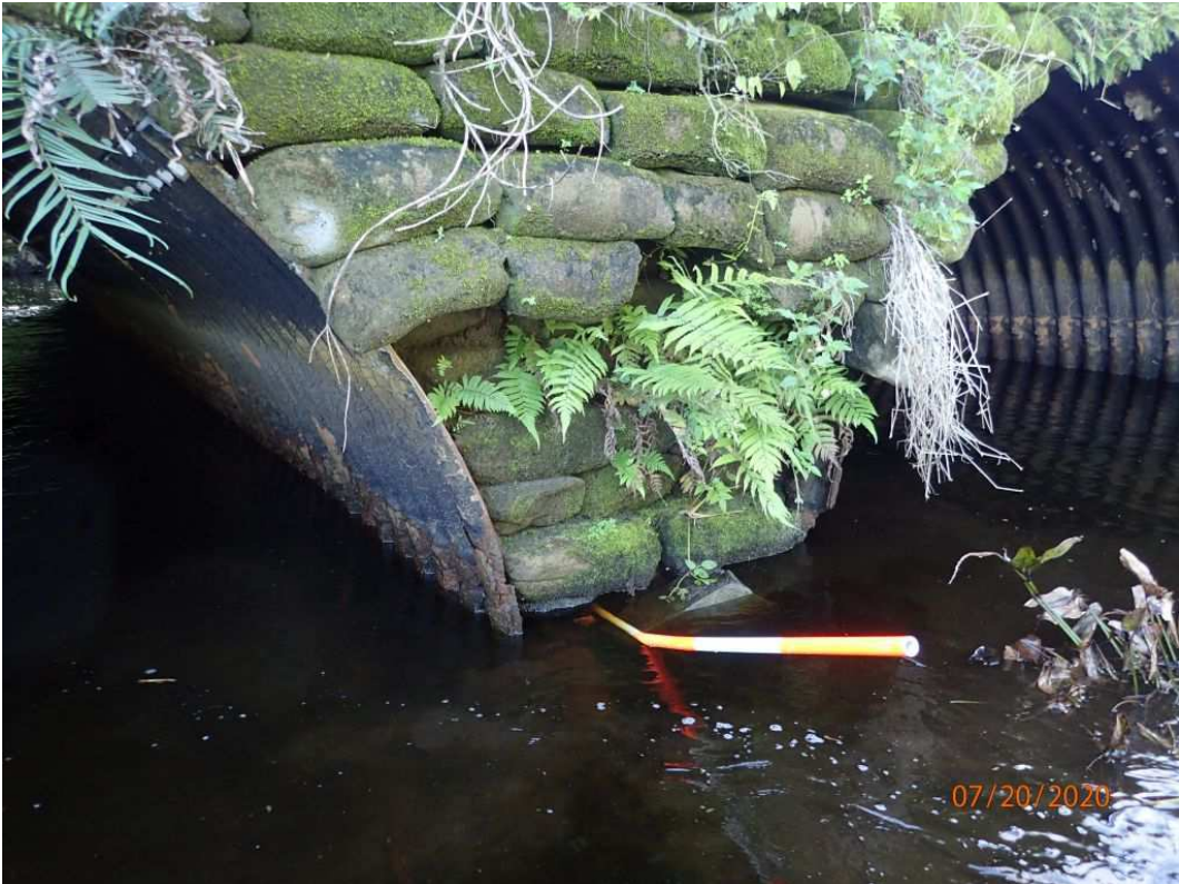
Photo 3: Element 8477: Missing bags from the west headwall between Pipes 3 and 4
