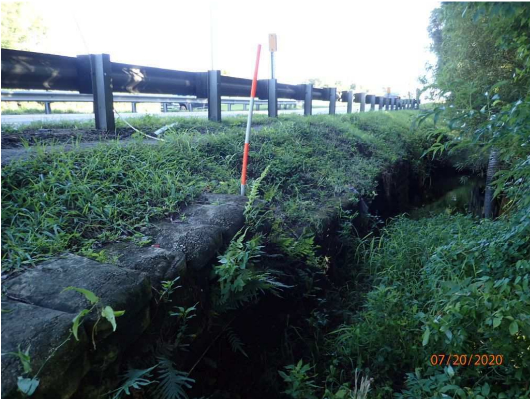
Photo 2: Element 8477: Sand cement rip rap bags missing from the east headwall at Pipe 1
