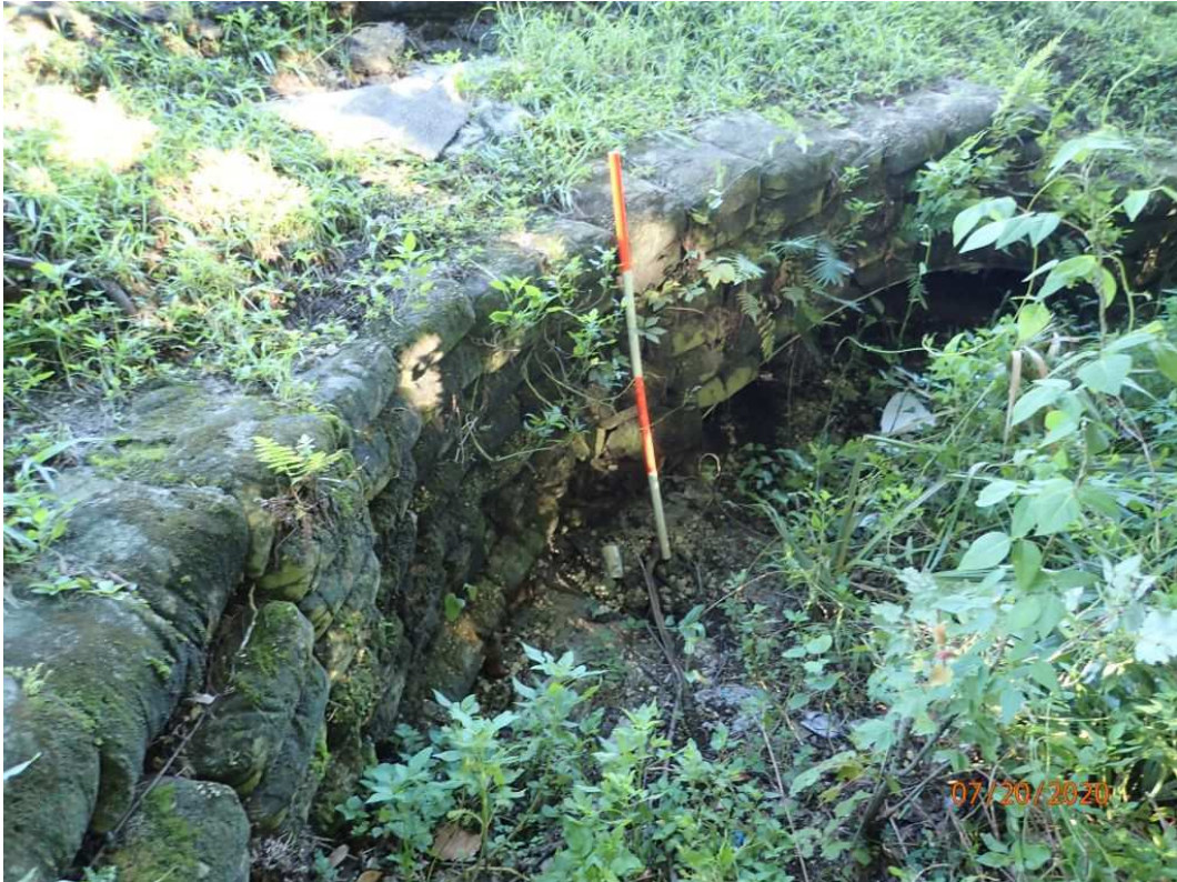
Photo 4: Element 8477: Settled sand cement rip rap bags in the east headwall over Pipe 1
