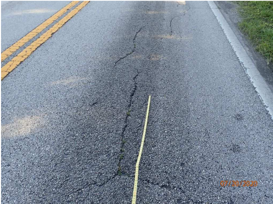
Photo 8: Inspection Notes: Crack in the asphalt surfacing over and approaching the structure
