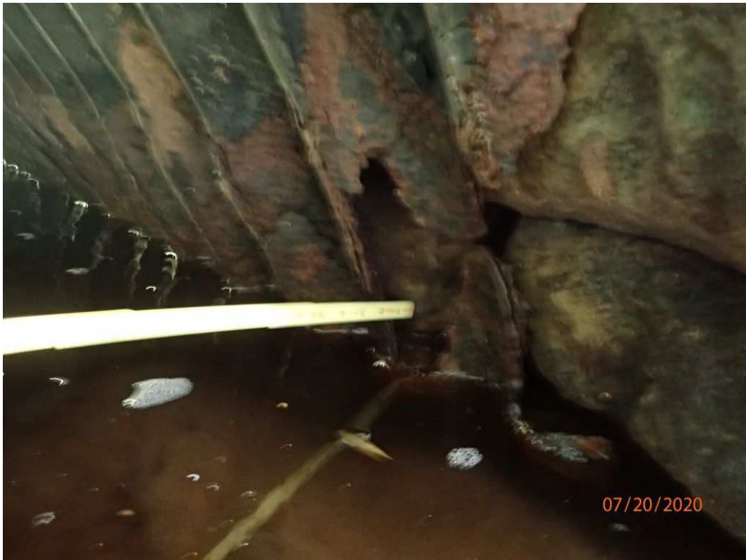
Photo 7: Element 240: Corrosion hole at the east end of Pipe 3
